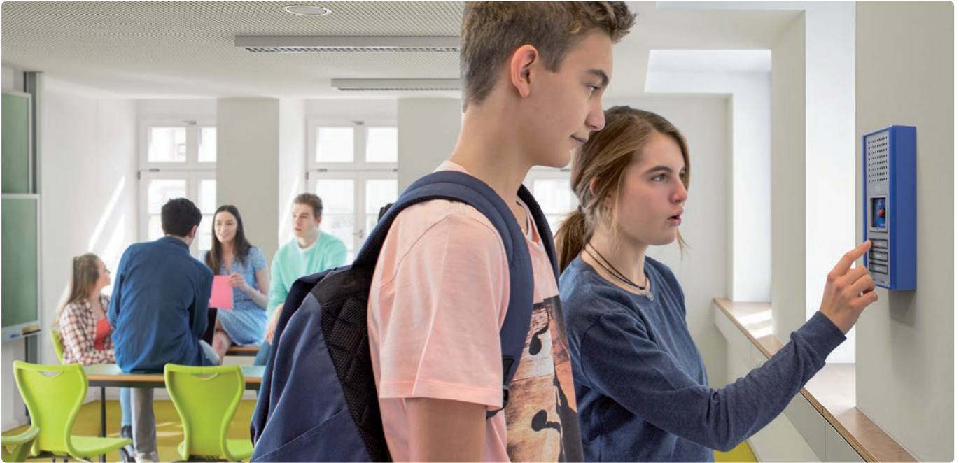
Intercom systems make it possible to communicate with the permanently occupied post and receive instructions in the event of an emergency.
